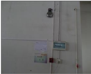
Photo of fire safety equipment 15 fire alarm.JPG
