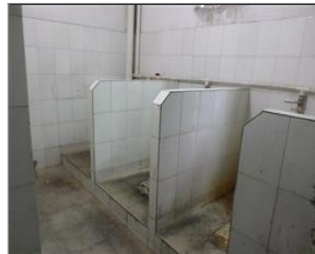
Photo of non-conformity NC6 no privacy doors.JPG
