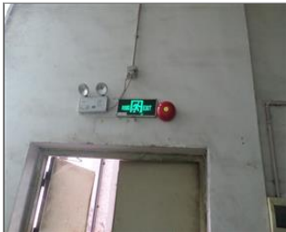
Photo of fire safety equipment 12 emergency light and exit indicator.JPG
