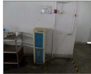
Photo of the inside of the main production hall 19 potable water.JPG
