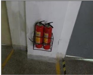
Photo of fire safety equipment 11 fire extinguisher.JPG
