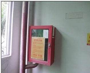
Photo of fire safety equipment 10 fire hydrant.JPG
